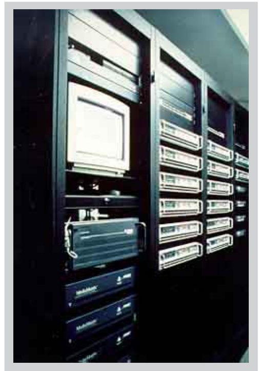
Main rack system
