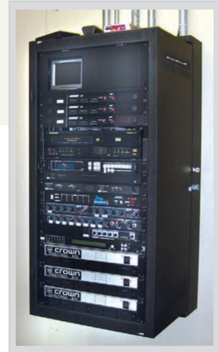
Equipment rack system
