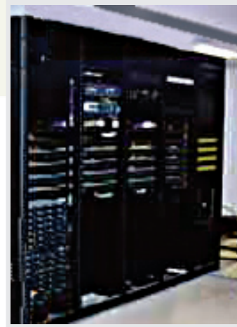
Main rack system
